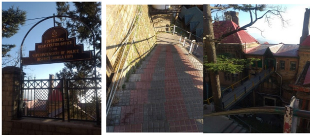
Stairs make it difficult for disables at the Superintendent of Police Office in Shimla. Ramps may be the alternative.
